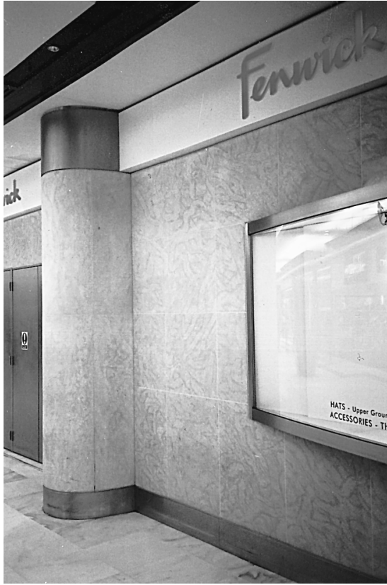
Fig. 2. Cladding on the groundfloor level of Fenwicks store, Brent Cross Shopping Centre. The slabs are 60 cm square.
